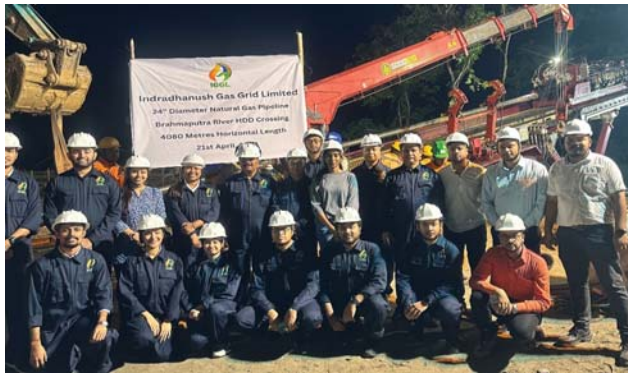
HDD crossing of length 4080 m of 24-inch Guwahati-Numaligarh pipeline across the Brahmaputra completed on 21.04.2023.
