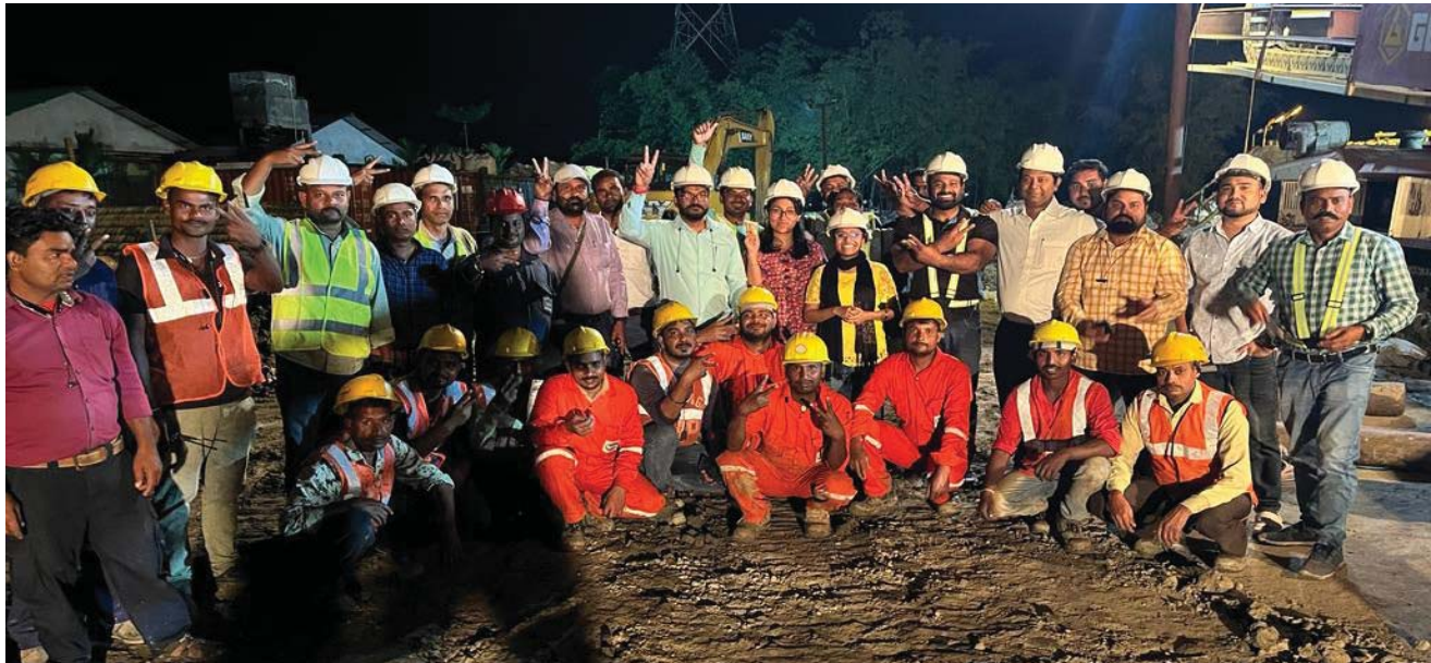
Successful completion of HDD of the Jia Bhareli river crossing of length 2.225 Km at Sonitpur, Assam on 09.04.2023.
