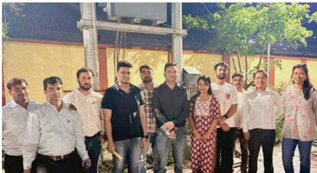
Charging of 160 KVA Transformer at DT, Panikhaiti
